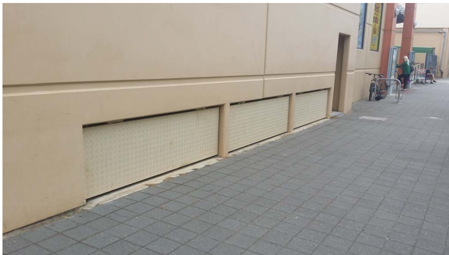
Flood gates under Mt Barker Central Shopping Centre
