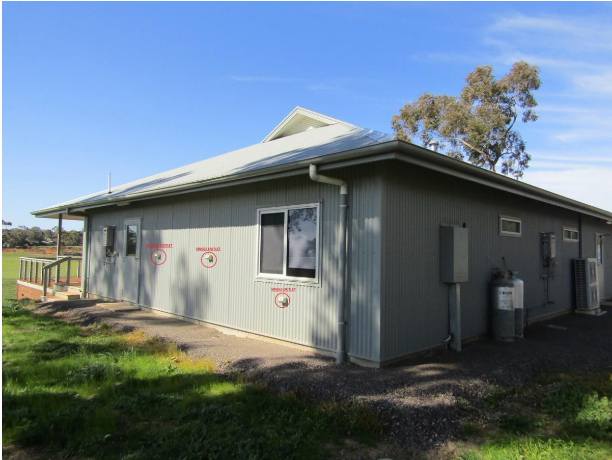
2 single and 1 double GPO on southern side of Polo Club Rooms
