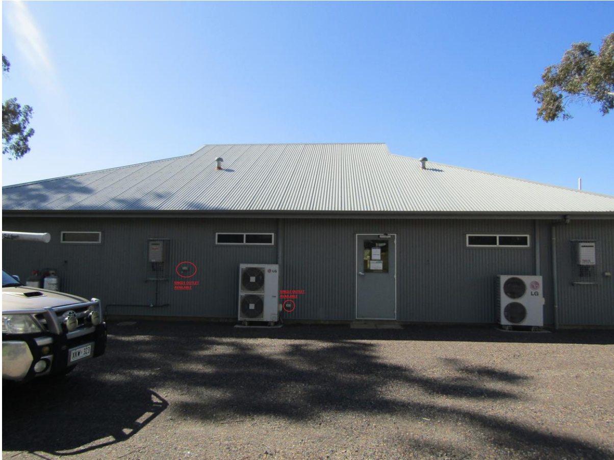
2 single GPOs at back of Polo Club Rooms
