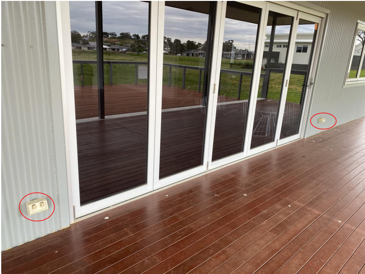
2 double GPOs on the deck area of Polo Club Rooms
