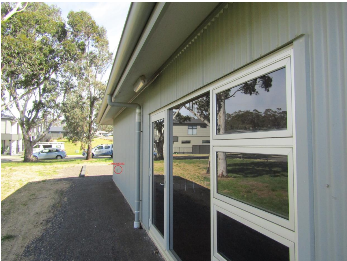
1 single GPO on northern side of Polo Club Rooms
