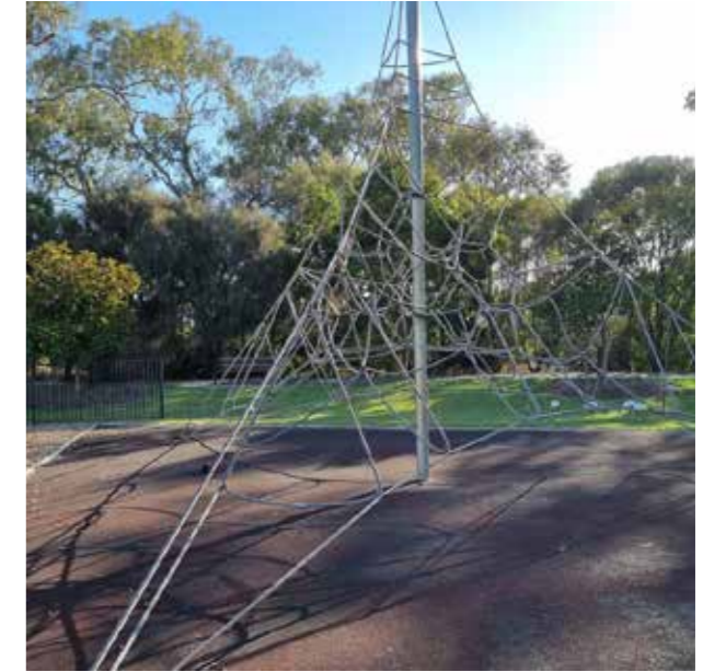
existing rope climb structure to be retained - rubber softfall to be replaced
