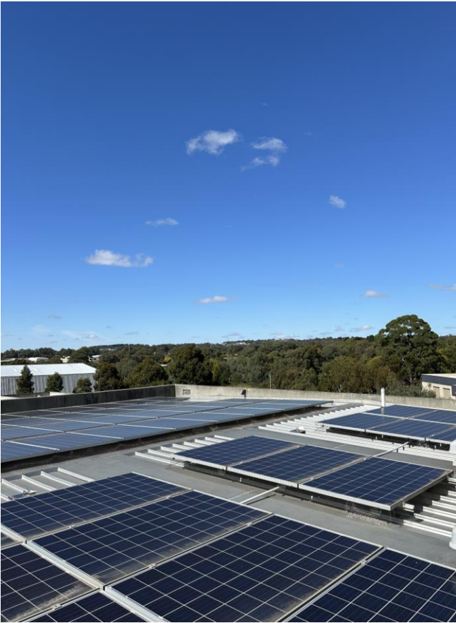
Figure 15: Civic Centre Solar PV System
